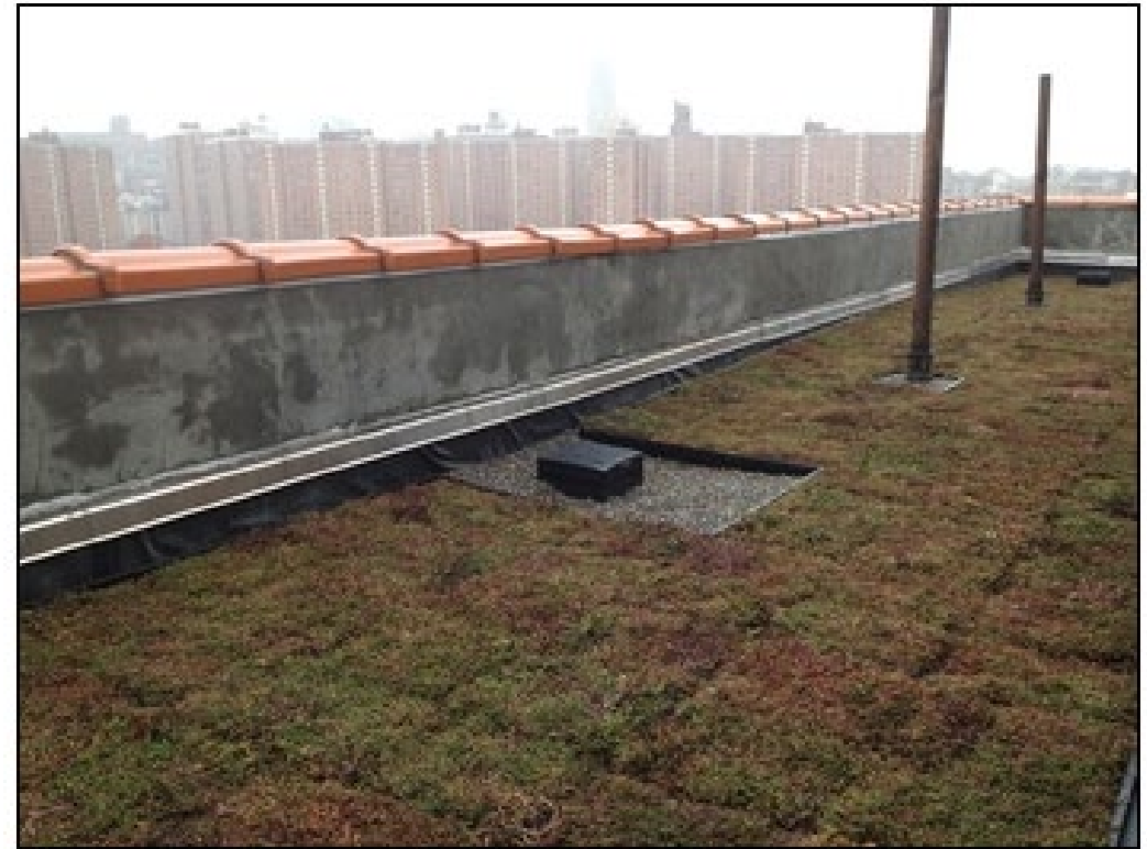
Green roof at Logan Gardens, a senior housing apartment building in Manhattan.
