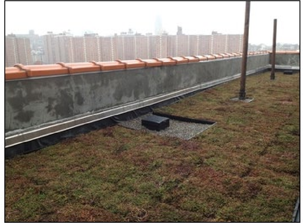
Green roof at Logan Gardens, a senior housing apartment building in Manhattan.
