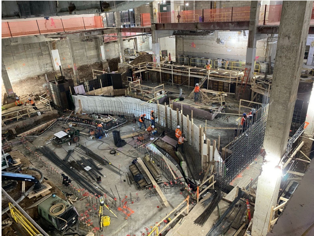
Rebar installation and concrete slab and footing pours ongoing in Large Venue.
