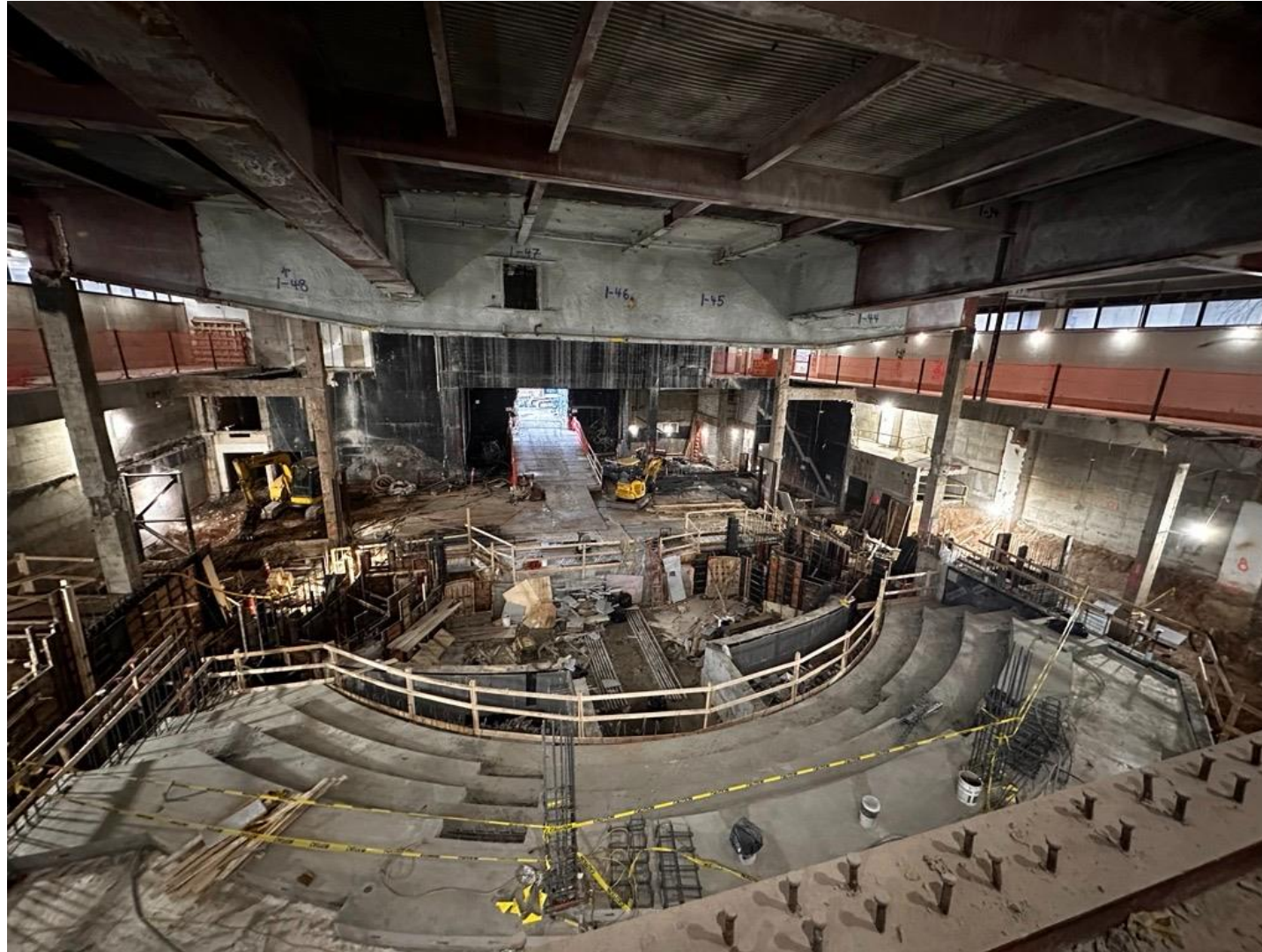
Concrete pour in balcony seating. Protections have been installed over the new stage slab in preparation for overhead structural demolition.
