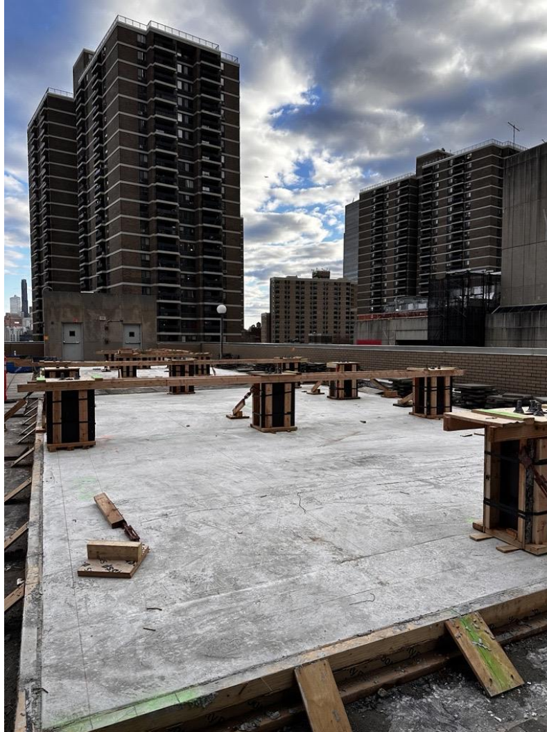
New concrete pad installation for new HVAC equipment on the 4 th Floor roof.
