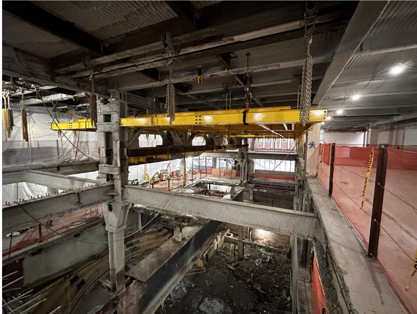
View of structural demolition in Large Venue from 2 nd Floor looking north.
